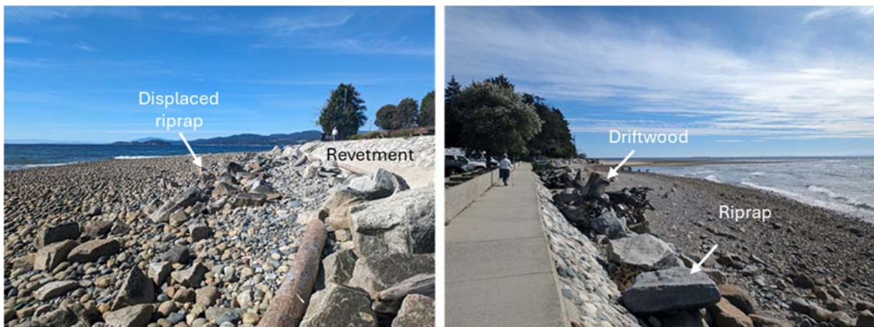
Photo 5 Davis Bay seawall and displaced riprap, indicative of high wave exposure. (left).
