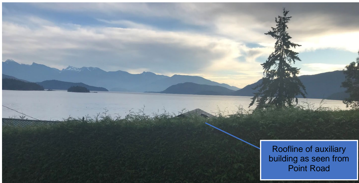
Figure 4 – View of roofline of partially constructed auxiliary building (subject of variance proposal) from Point Road
