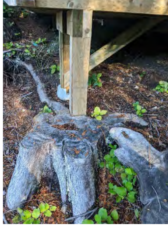
View of the footings, several footings are placed directly on the ground/stumps or concrete deck blocks.
