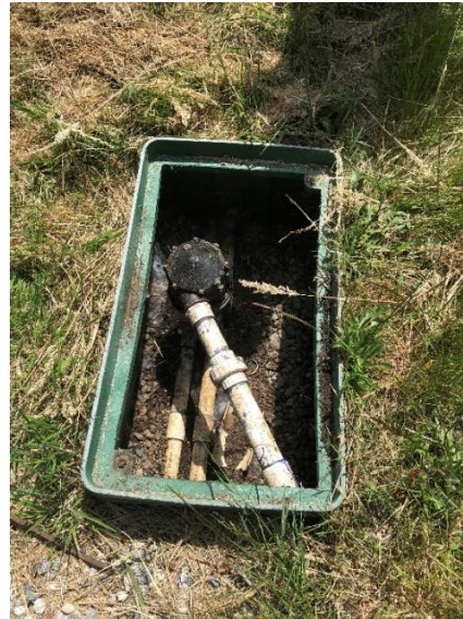
Figure 10 – Distribution Box to Zone 1 of the RSF
