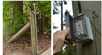
Existing water and power access for large picnic table to be upgraded.
