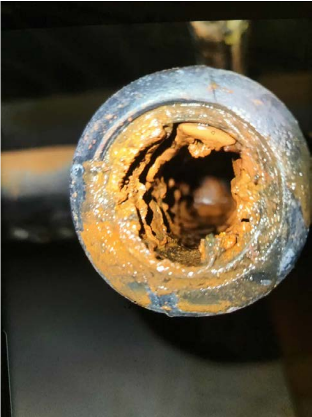
Photo – Mechanical Room
