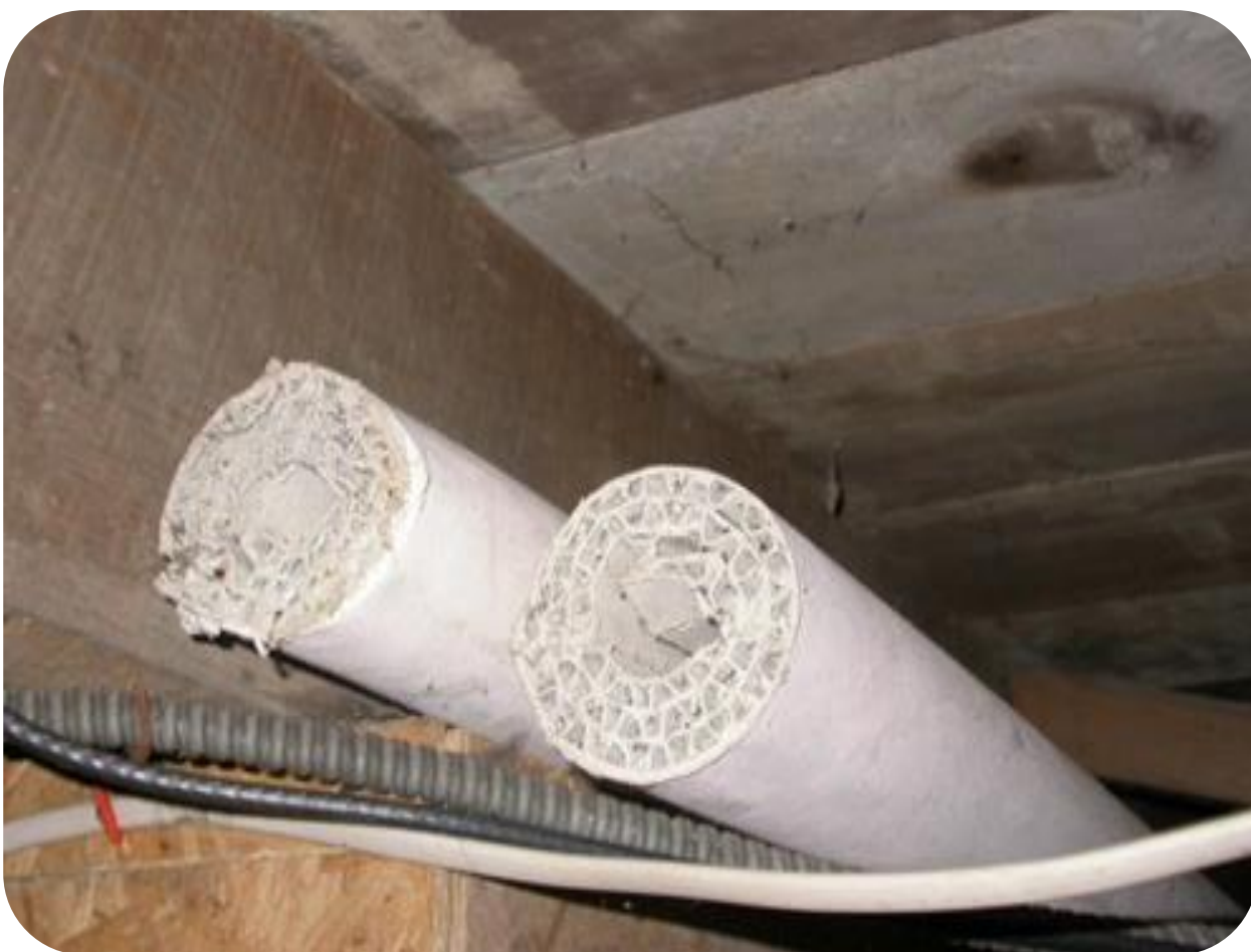
Corrugated Pipe Insulation
